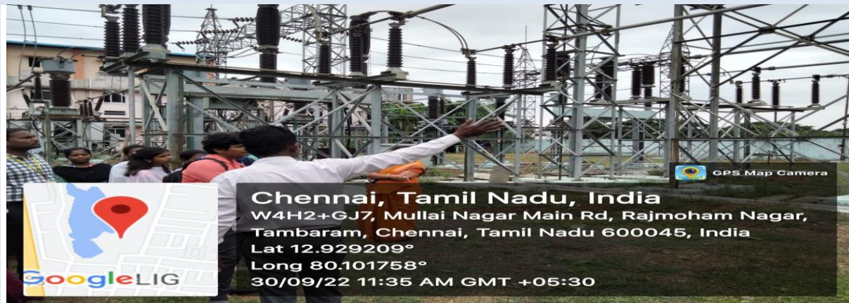
110/33-11KV Power distribution to consumer end at various loads
